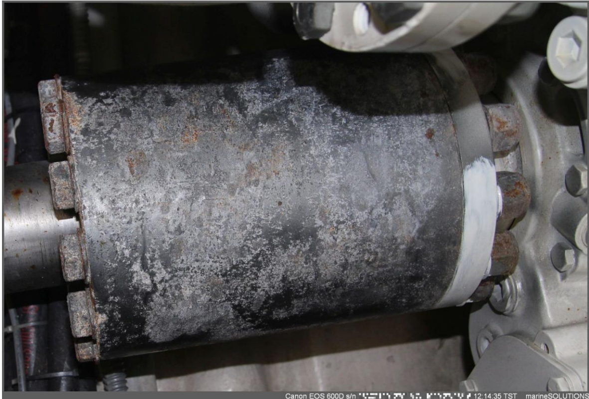
Surface corrosion of the port shaft coupling and its bolts.
