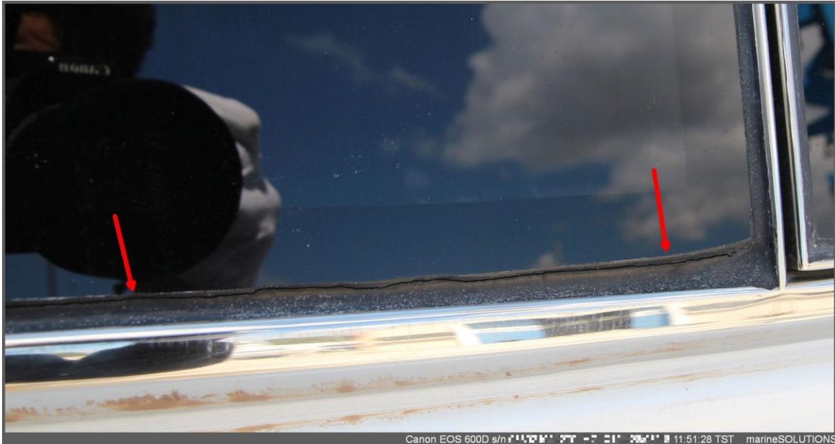
Detachment at the starboard side window mastic.
