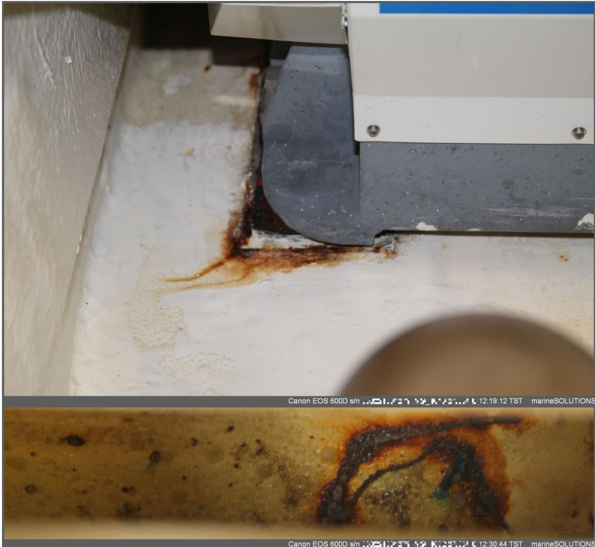
Top: Corrosion products leaking from one ARG unit's mount. Below: Salt crystals and a heavily corroded metal part located in between both ARG units.
