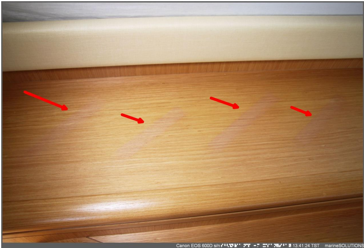
Four frame marks on the counter top at the side of the dinette area.
