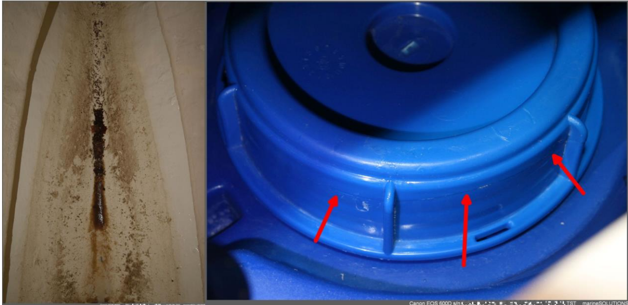
Left: Living quarter bilges tidemarks due to the leaking fresh water tank. Right: The crack on the cap of the fresh water tank.
