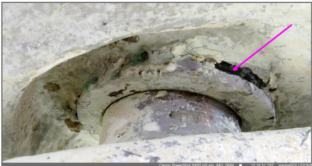
Above: Deteriorated sealant around the rudder shaft's lower bearing
