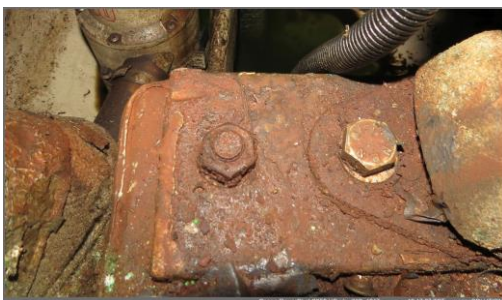
Right: One of the mount of the engine which is heavily corroded
