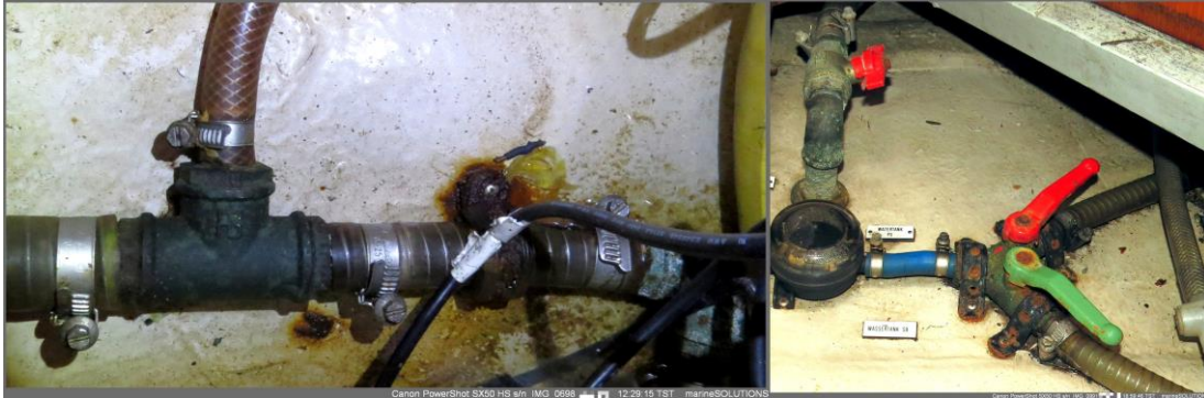
Above left: Equipment in the forward hallway bilge. Above right: Equipment in the galley's forward bilge
