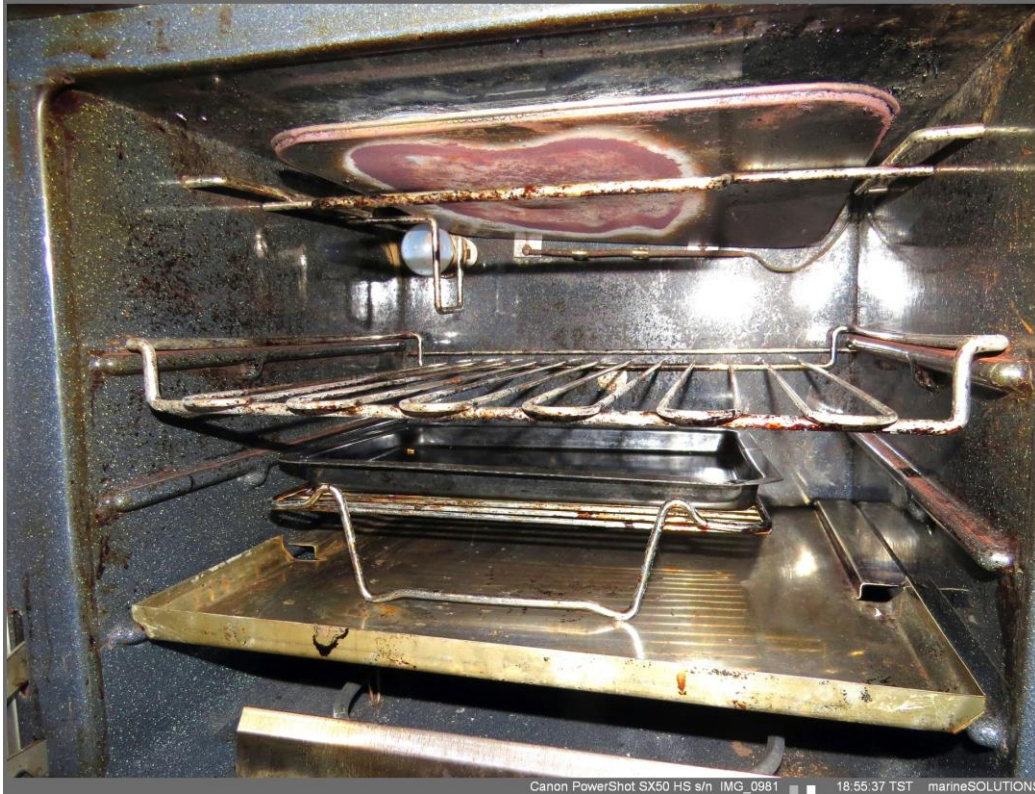
Above: The condition of the oven/hob
