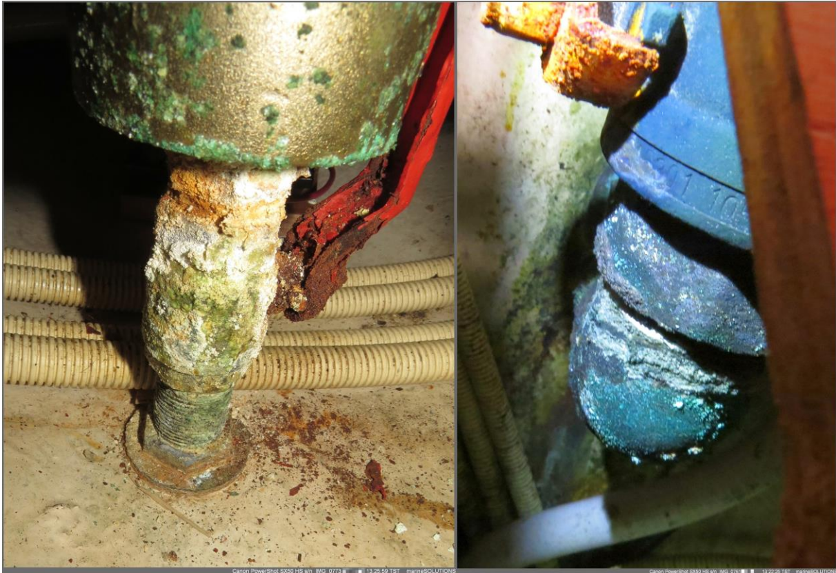
Above: Examples to the corroded seacocks
